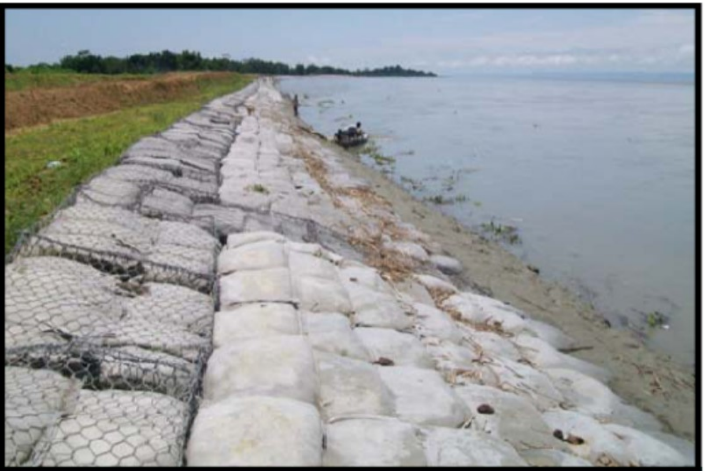
Condition of Geotextile Bags & River Bank After Flood
